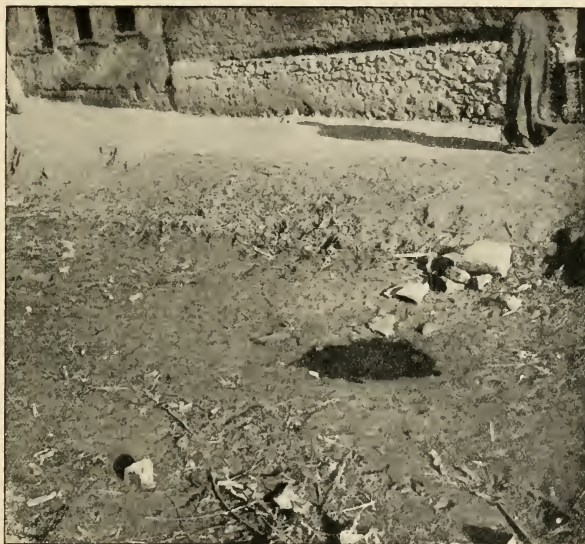
FIG. 33.—The bed of the Marg Canal in the village during a summer rotation.
